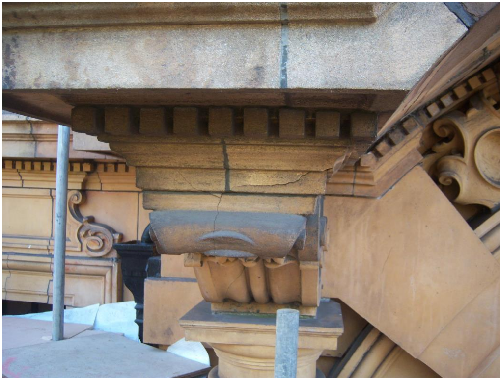
Fractures evident throughout both corbels in all directions
